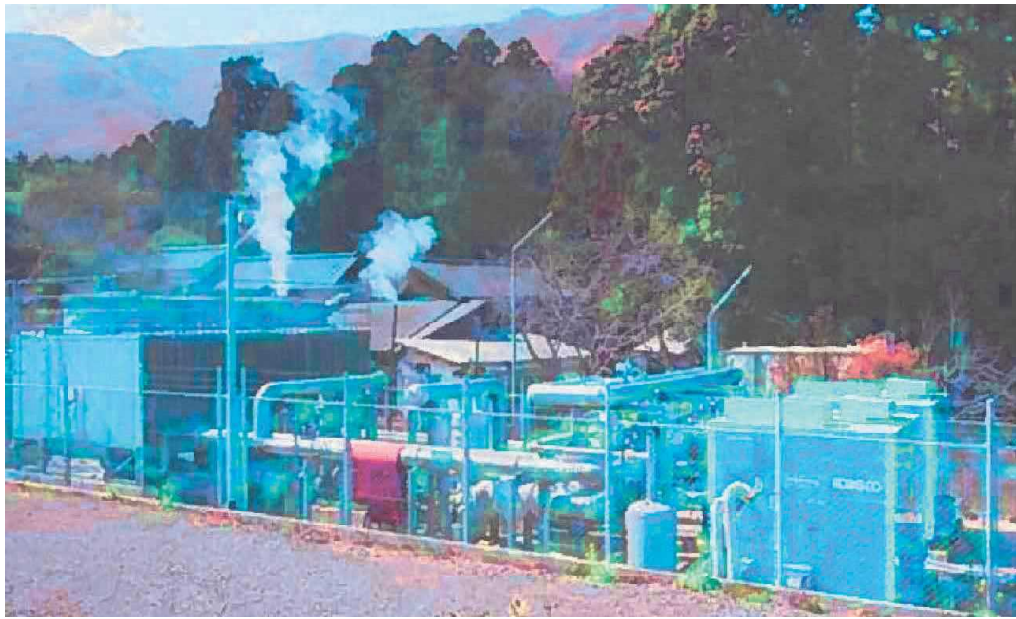
Figure 3-8 Yuyama Geothermal Power plant
