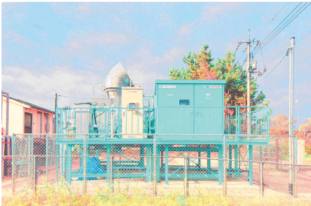
Figure 3-9 Yurihama Geothermal Power plant
