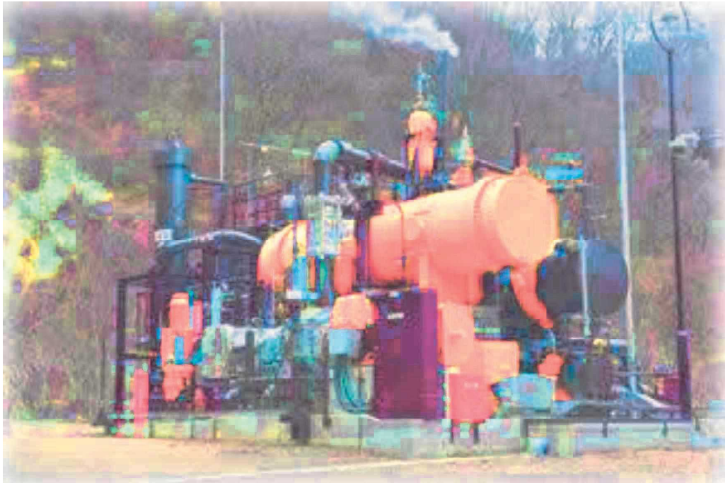
Figure 3-10 Tsuchiyu Onsen #16 Source Binary Power plant
